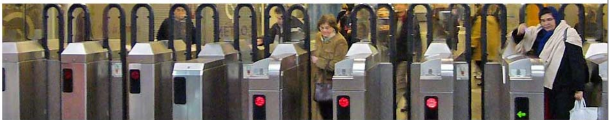
Automated ticket control. Milan Metro, Italy, 20
