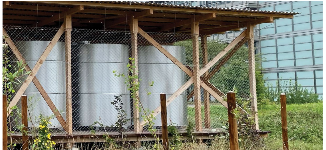
10 MWh seasonal energy storage pilot plant at ETH Hönggerberg campus
