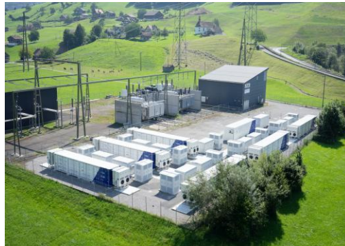
Battery Energy Storage
