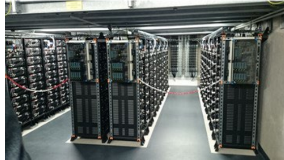
Electrical Energy Storage
