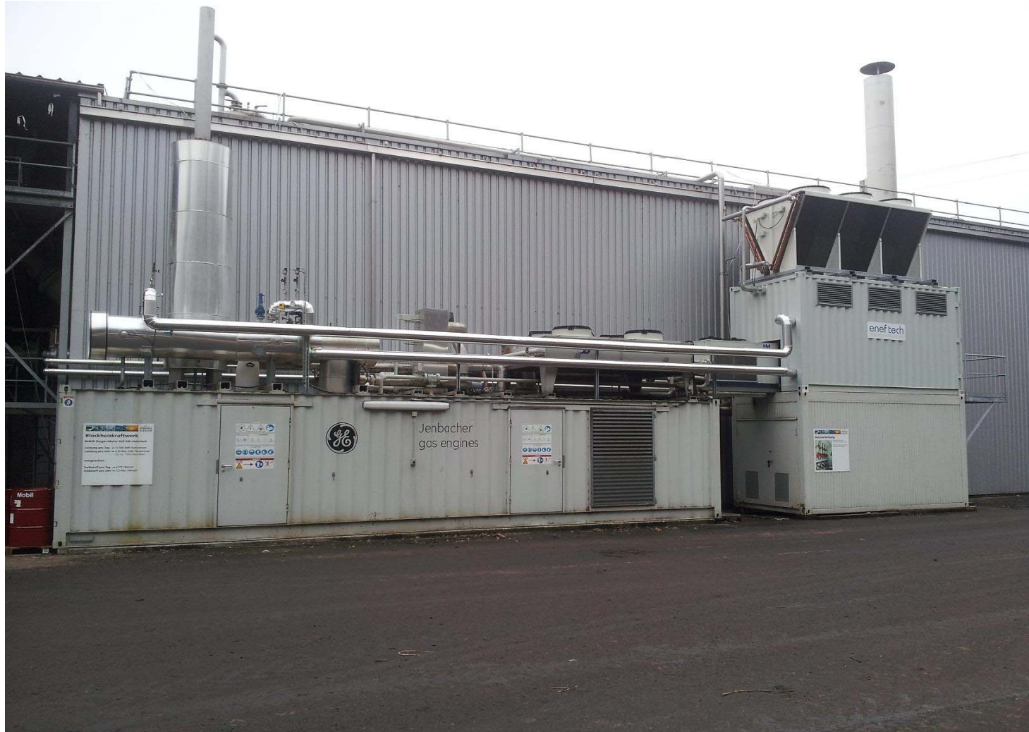
500kW biogas engine, 30kWe ORC unit in Klingnau, Eneftech 2013
